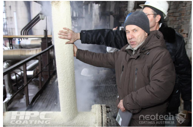
FIGURE 5: HBC IS SAFER FOR PERSONNEL WITH 30 MM OF COATING APPLIED TO 470+°C STEAM PIPES TO 40°C
