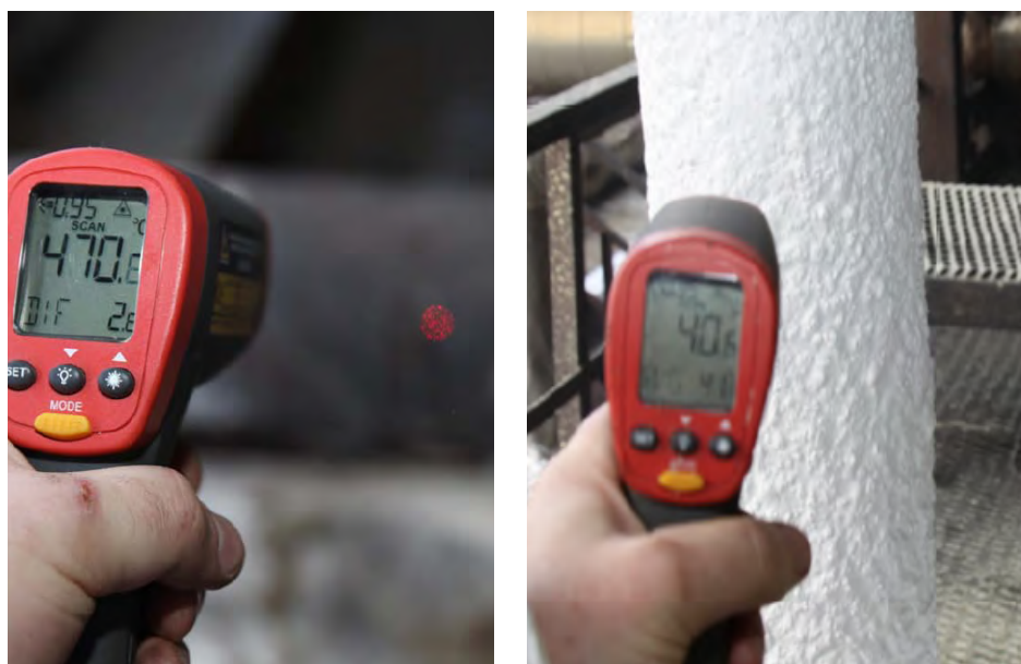
FIGURE 1: STEAM PIPE AFTER 30MM OF THICK CLOSED FILM CERAMICS TIC ON 550C PIPE DOWN TO 40°C
