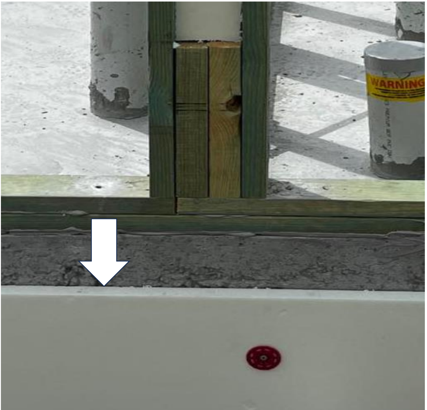
A clearer view of the insulation relative to the slab edge with XPS (arrow) exposed.
